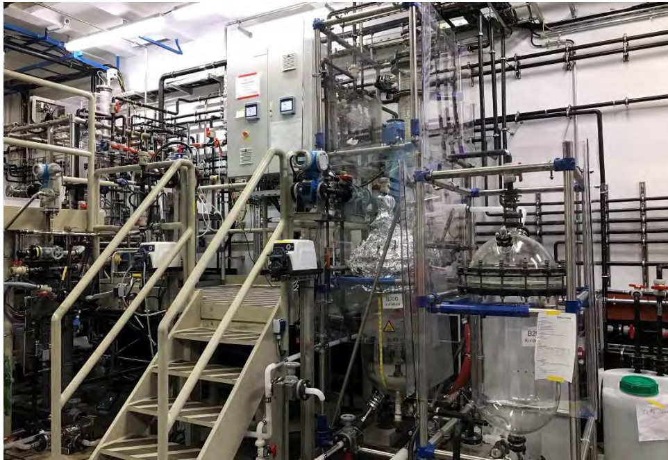
Figure 3 – Photograph of the Pilot plant showing Reductive leach system and Lithium evaporation system.
