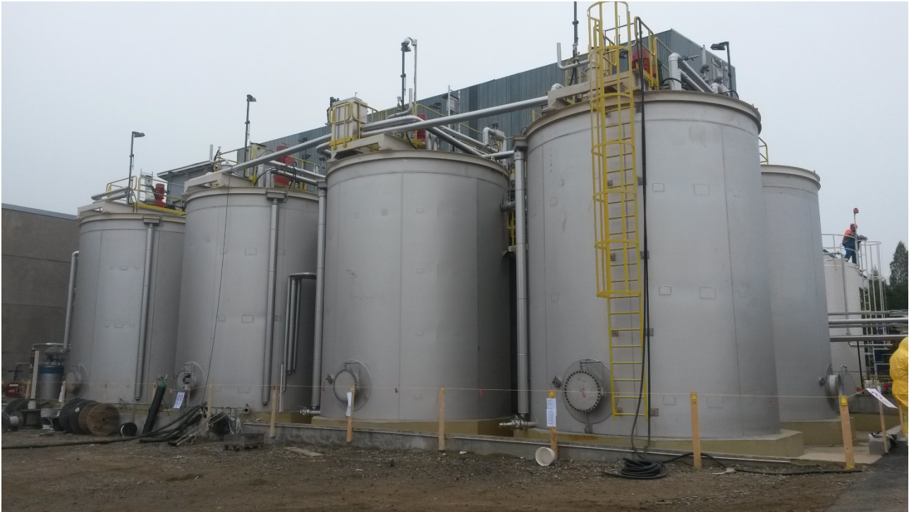
Figure 23: The bioleach reactors at the Mondo Minerals nickel sulphide plant (37)
