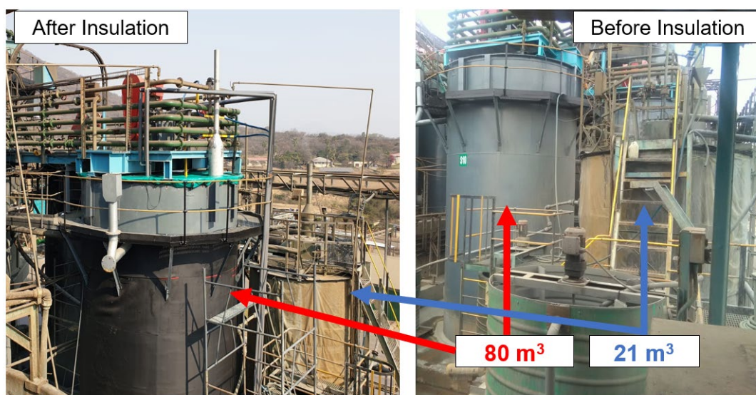
Figure 12: Views of the engineering (21 m 3 ) and demonstration (80 m 3 ) scale thermophile reactors
