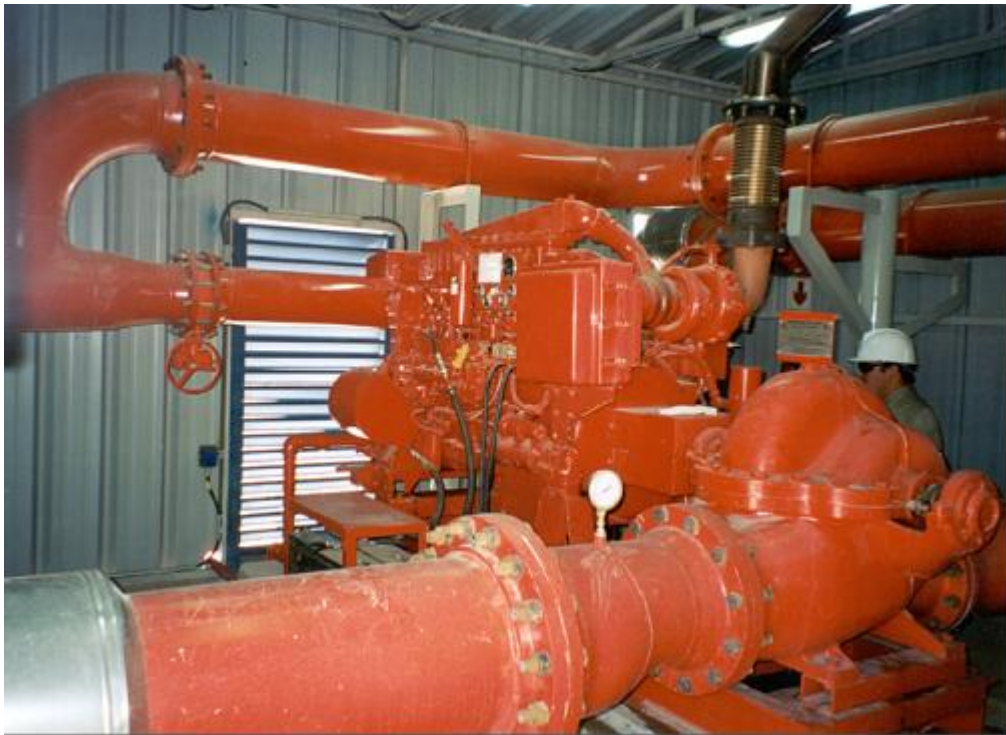
Figure 7. Cerro Mocho Pump. This is capable of 320 l/s (5,100USgpm) and is connected to the back up water supply.
