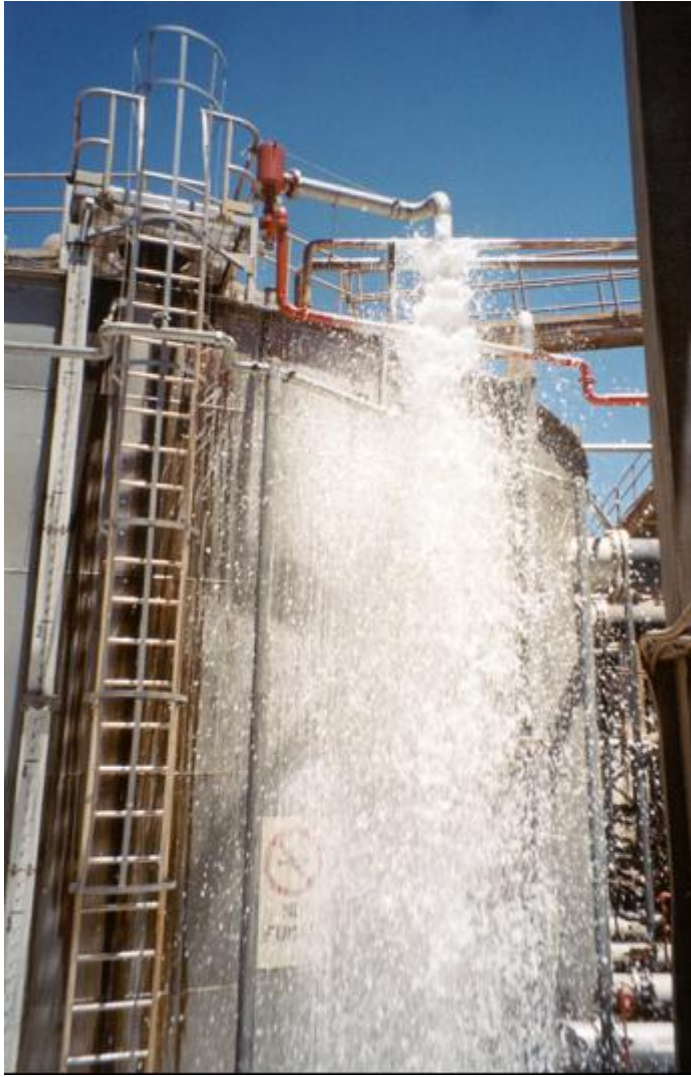
Figure 12. Discharge test for the low-expansion foam in the organic surge tanks in the tank farm. The foam generator has been turned around and a test piece attached to discharge the foam onto the ground. Tests such as these need to be done at the frequencies specified in NFPA 25 as a minimum requirement.
