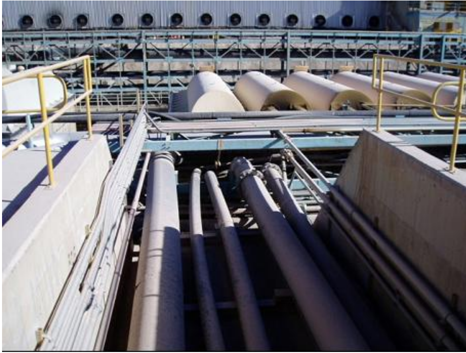
Figure 2. An example of a deep pipe trench connecting the mixer/settler train with the tank farm. A wall needs to be built here to prevent spilt organic liquors flowing into the tank farm. This trench, together with the trenches around the mixer/settlers, has sufficient capacity to hold the potential spillage if all of the pipes are ruptured by fire and hence it is not proposed to divert the spillage to another location.
