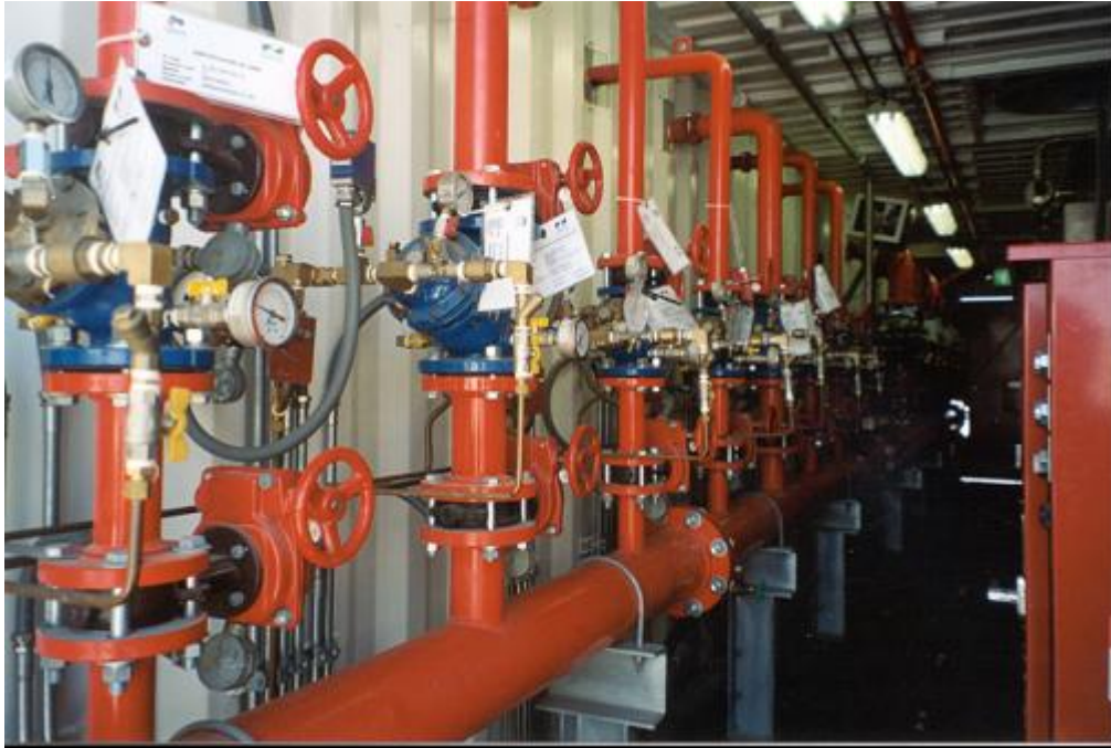
Figure 10. Lo-Expansion foam valves in the FSCC.
