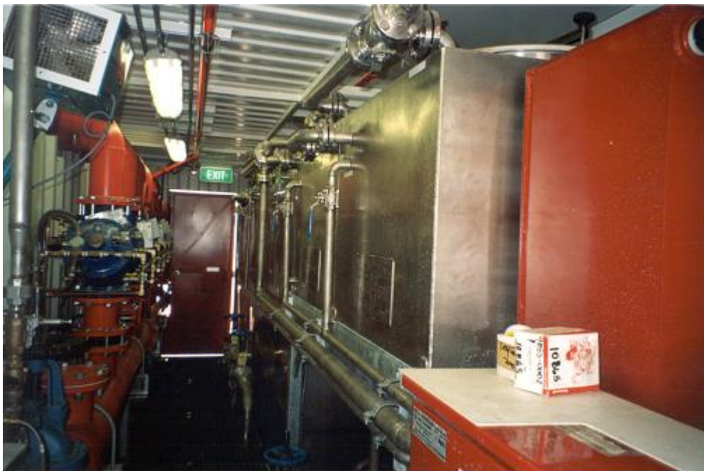
Figure 9. Interior view of one end of the FSCC. The storage tanks for the low-expansion and hi-expansion foams are shown on the right and the bank of deluge valves are shown on the left.
