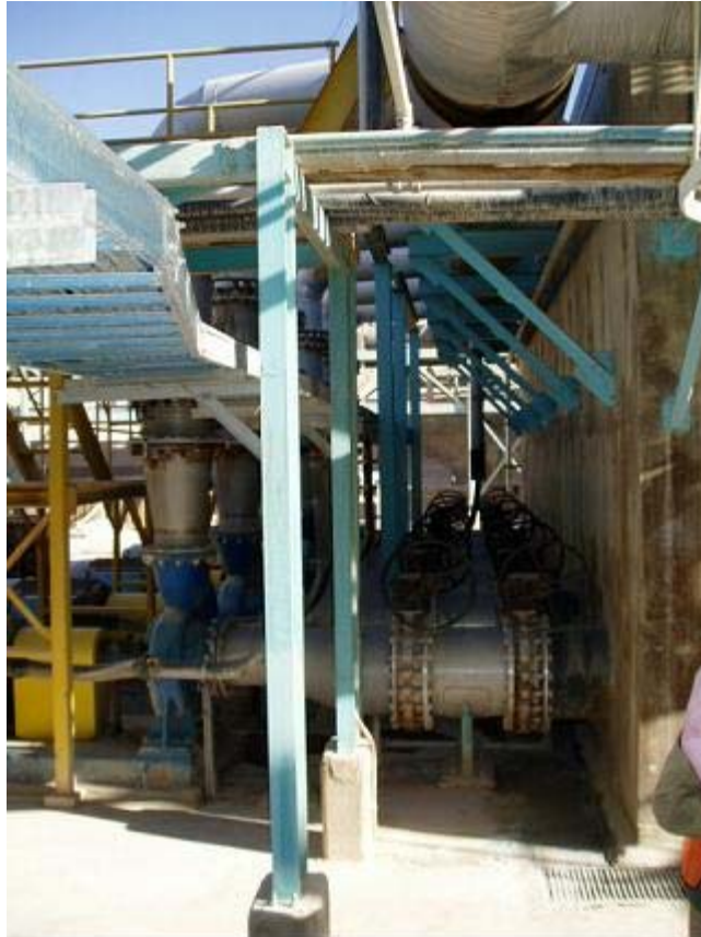
Figure 5. Arrangement of the organic pumps at the surge tank. Note the use of stainless steel for all pipe connections including the expansion/ isolation bellows on the discharge lines of the pumps. The stainless steel piping also extends up to the top of the surge tank.
