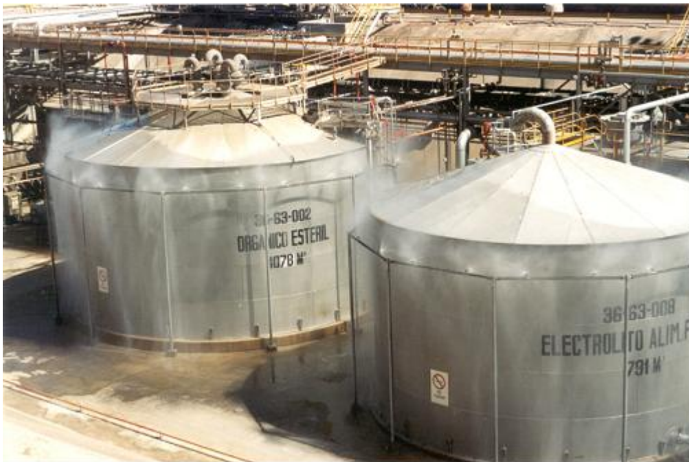
Figure 11. Discharge test of the tank farm exposure sprinklers. At Zaldivar all tanks are from stainless steel and the water provides cooling in the event of a fire to maintain the structural integrity of the tanks. Low-expansion foam is discharged into the interior of the tanks.
