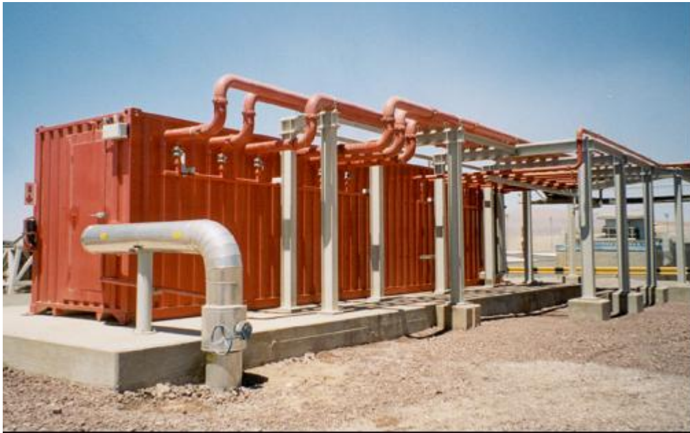
Figure 8. Rear view of the container housing the Fire System Control Centre (FSCC). All of the foam, foam valves and pumps, and deluge sprinkler valves are housed in this container together with the main control panel for the fire protection system.
