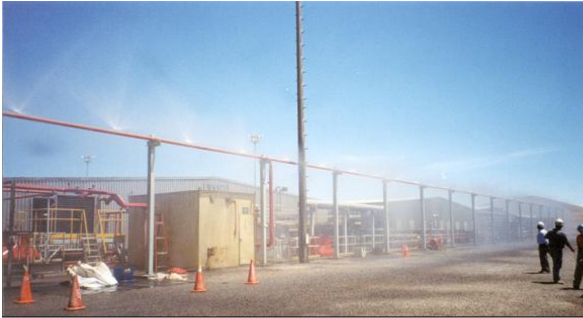
Figure 15. Discharge test of the water curtain that has been installed between trains B and C. This acts as a radiant heat barrier between the two trains effectively dividing the SX plant into two halves. The distance between these two trains is approximately 15m which is insufficient to prevent radiant heat from a major fire in one half from adversely affecting the integrity of the plant in the other half, particularly the HDPE piping.
