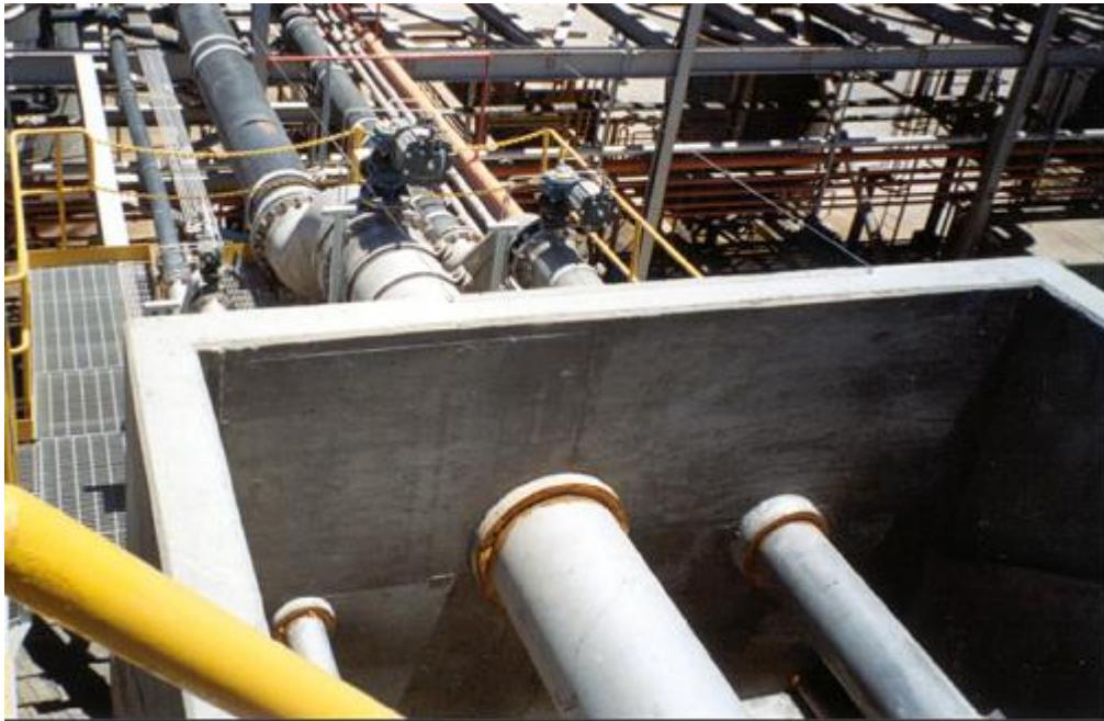
Figure 6. Retaining wall at the end of the trench for pipes from mixer/settlers. Note the stainless steel spool pieces penetrating the wall and the automatically closing isolation valves on all pipes on the downstream side of the walls. The separation of the SX plant into manageable areas through the installation of containment walls results in lower costs for the fire protection equipment and a much high likelihood of success in limiting the extent of the damage from a fire.
