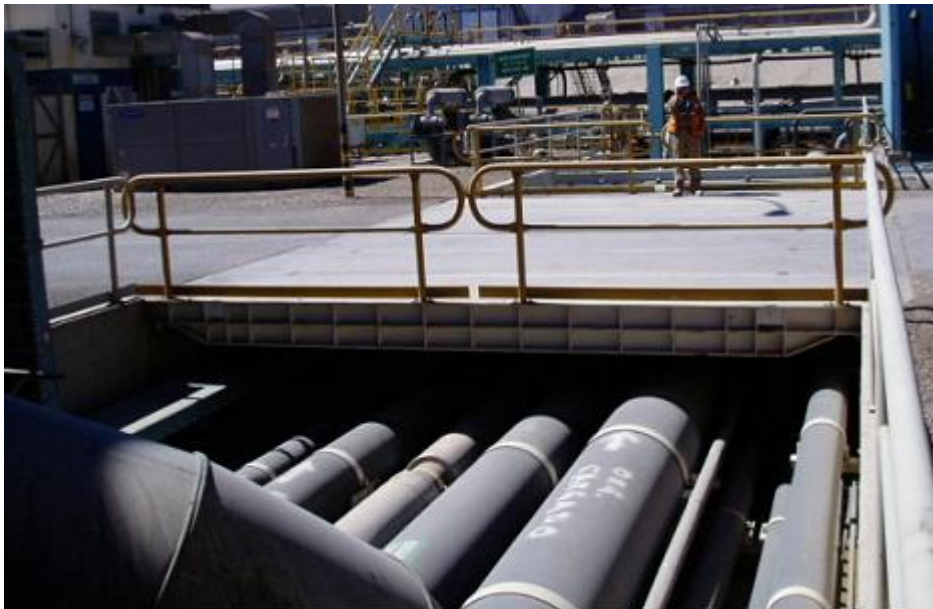
Figure 3. An example of a shallow pipe trench with a much higher density of HDPE piping. At this SX plant the pipes are almost at ground level at the mixer/settlers and it is proposed to install underground pipe drains that take the spilt liquor away to a disposal pond. A retaining wall at the junction of the trench with the tank farm is also to be installed.
