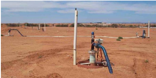
(ISL Wellfield, Beverley Operation, Heathgate Resources, South Australia)
