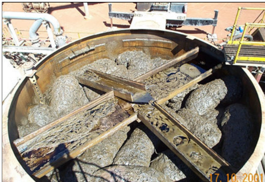
Figure 5: Loaded Organic Coalescer ready for cleaning
