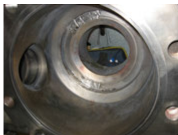
Leak Path on Seat Land
