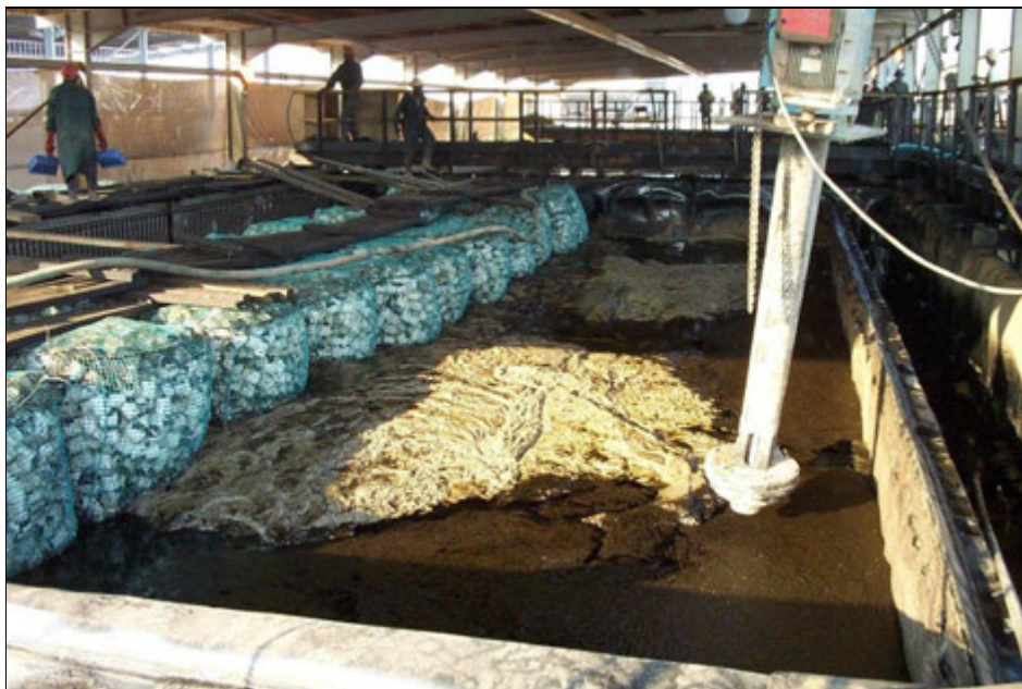
Figure 1: Severe Crud Infestation in a Settler
