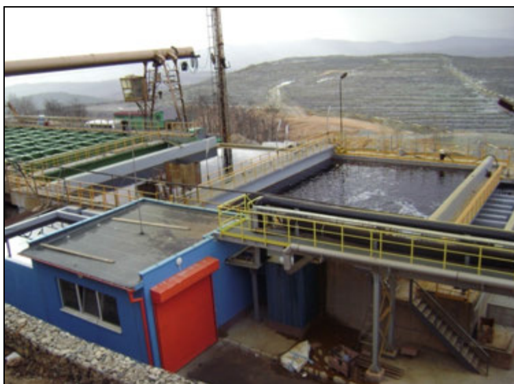
Figure 8: Reconstructed Cementation Cells and PLS and Raffinate Tanks.
