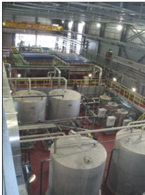
Figure 5: Tankfarm and Electrowinning.
