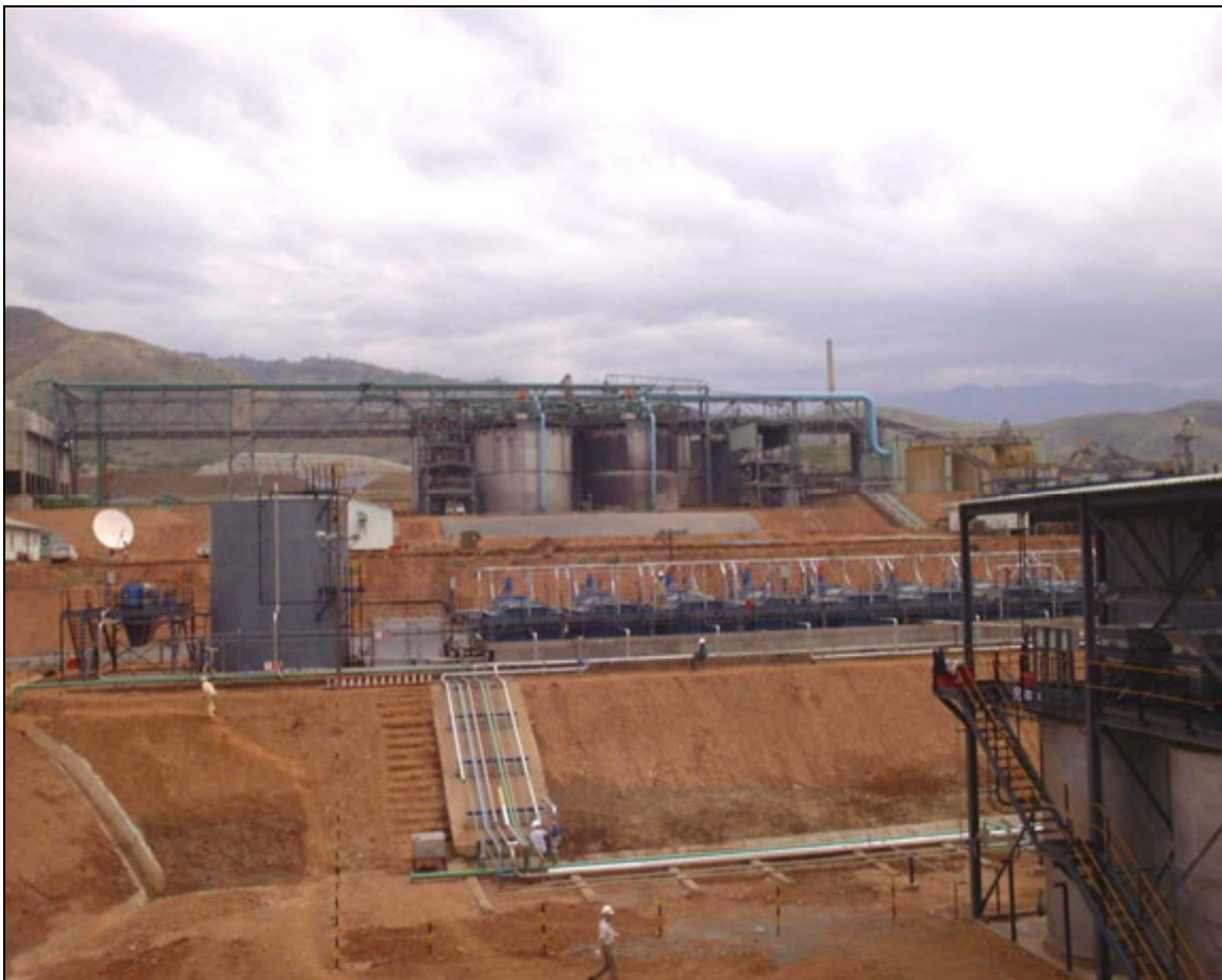
Figure 5: KCCL Bioleaching Plant
