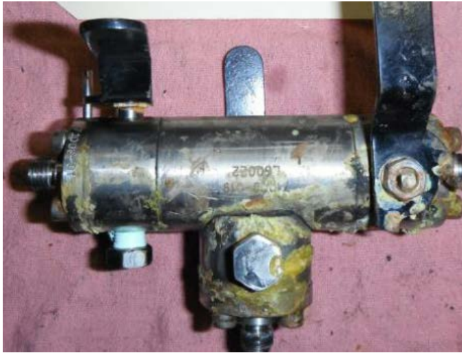
Ball Valve Body Leakage
