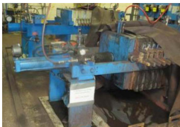
Figure 25: Demonstration Plant Filter
