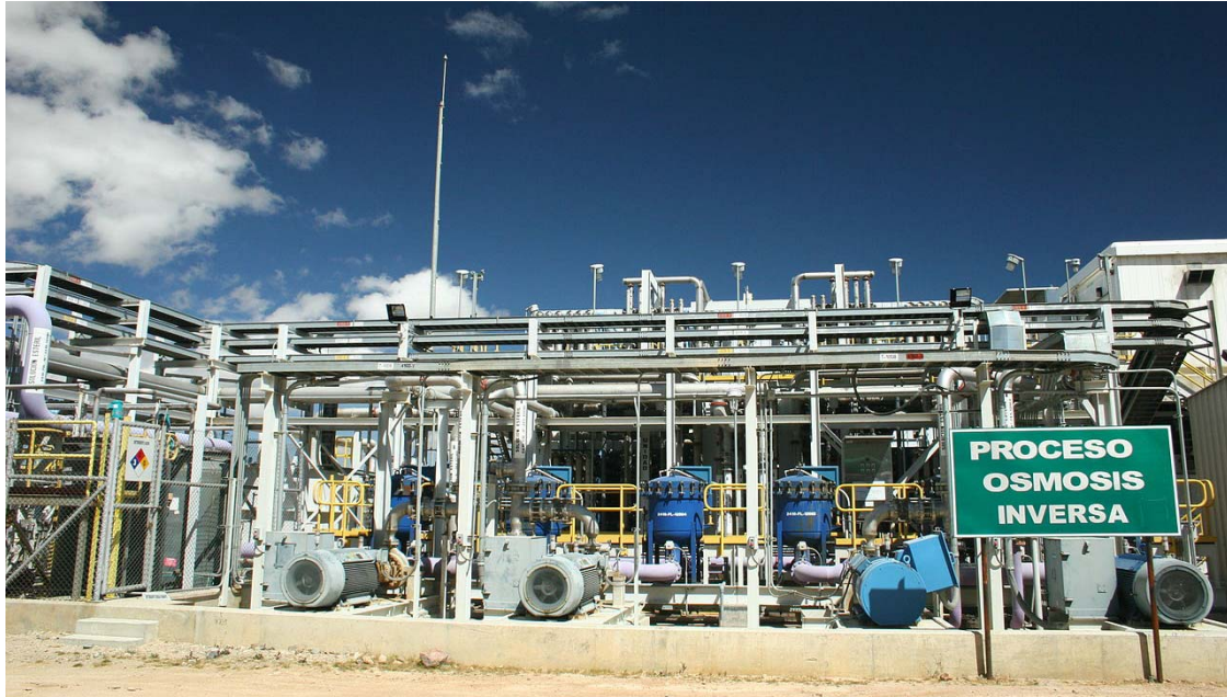
Figure 3: Yanacocha 2004 reverse osmosis water treatment plant (after Elbuenminer) (8)
